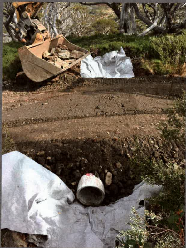
Construction of a fauna crossing on Happy Valley ski run, Perisher. (Photo: Tanya Bishop, Perisher ski resort)
